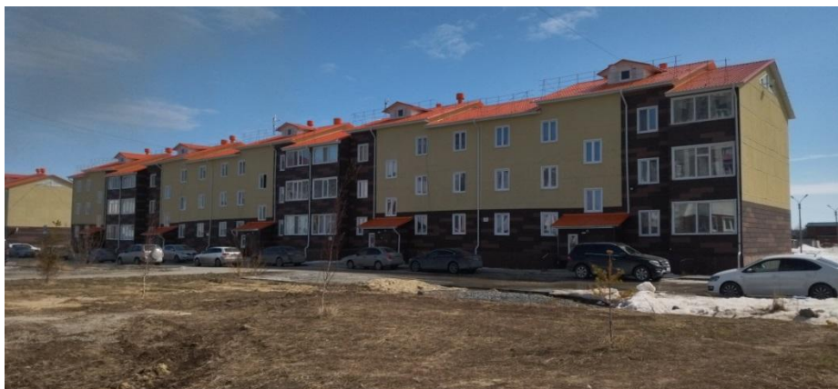
Figure 1: A new framed residential building that has undergone significant deformation due to the thawing of soils in permafrost conditions
