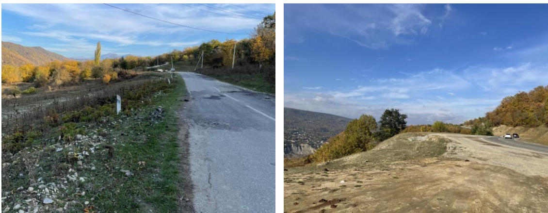
Figure 3: Landslide processes near the Nozhai-Yurt - Sayasan highway
