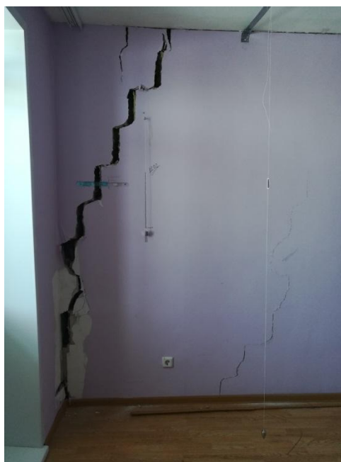
Figure 1: deformation of a building in arctic conditions due to uneven settlement of the "soil-building" system
