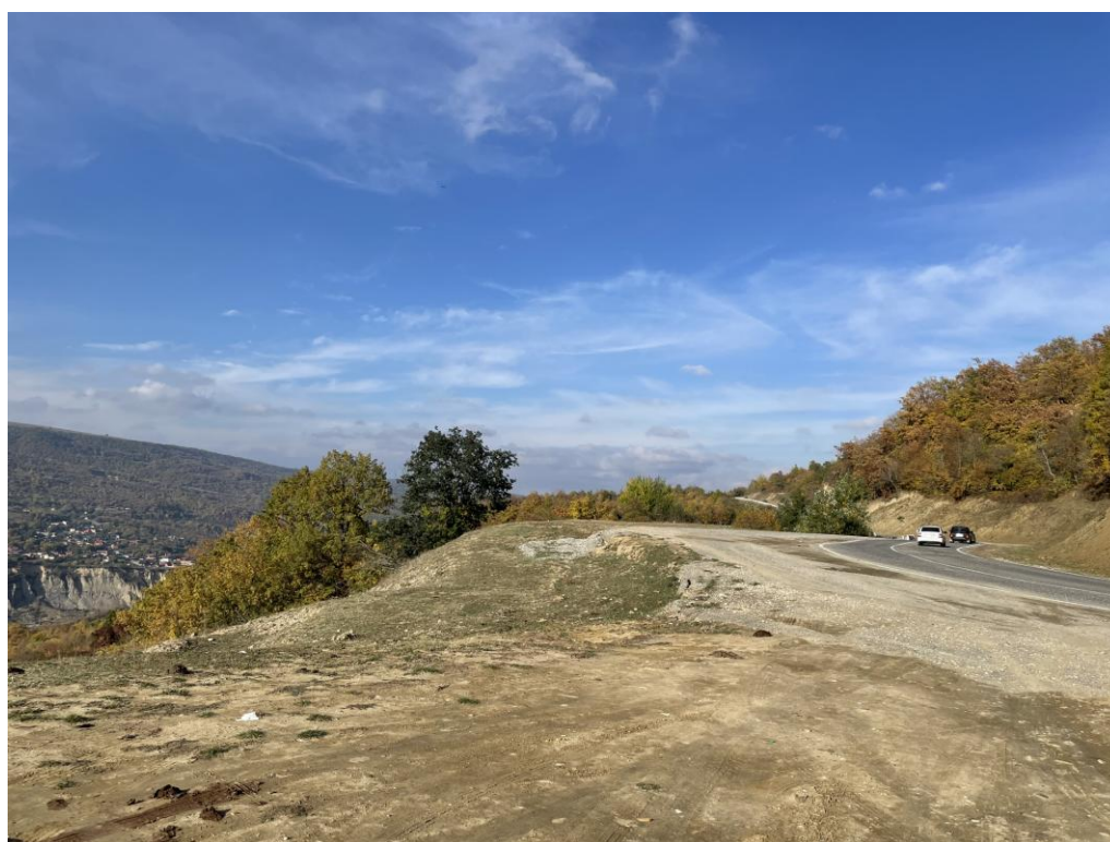
Figure 2: Landslide processes near the Gendargen-Shunoy road
