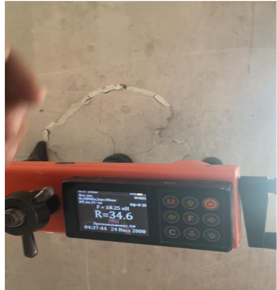
Picture 2: Shear test method (crack formation)
