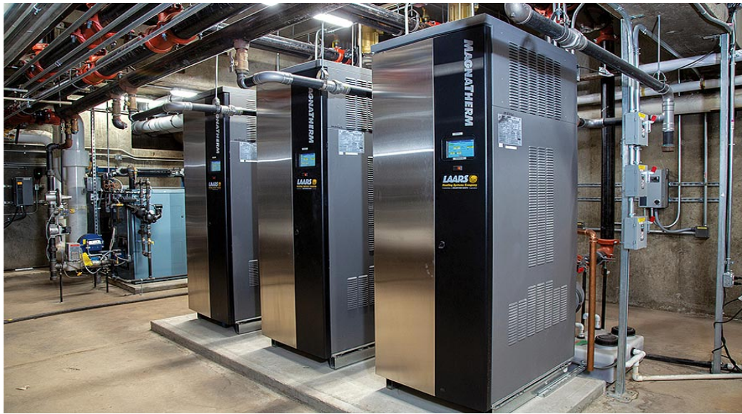
Figure 5: Parallel Boiler Cascade System
