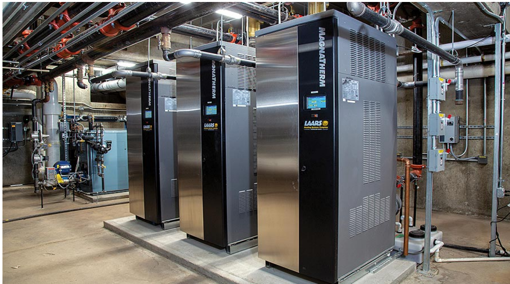
Figure 5: Parallel Boiler Cascade System
